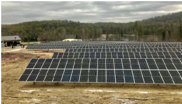
Hanover's Grasse Road Solar Farm
