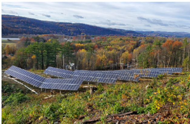
Charlestown Solar Array
